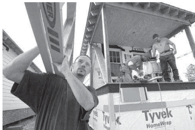
A work crew constructs a house that the Southern Mutual Help Association helped finance. Photo courtesy of SMHA.
